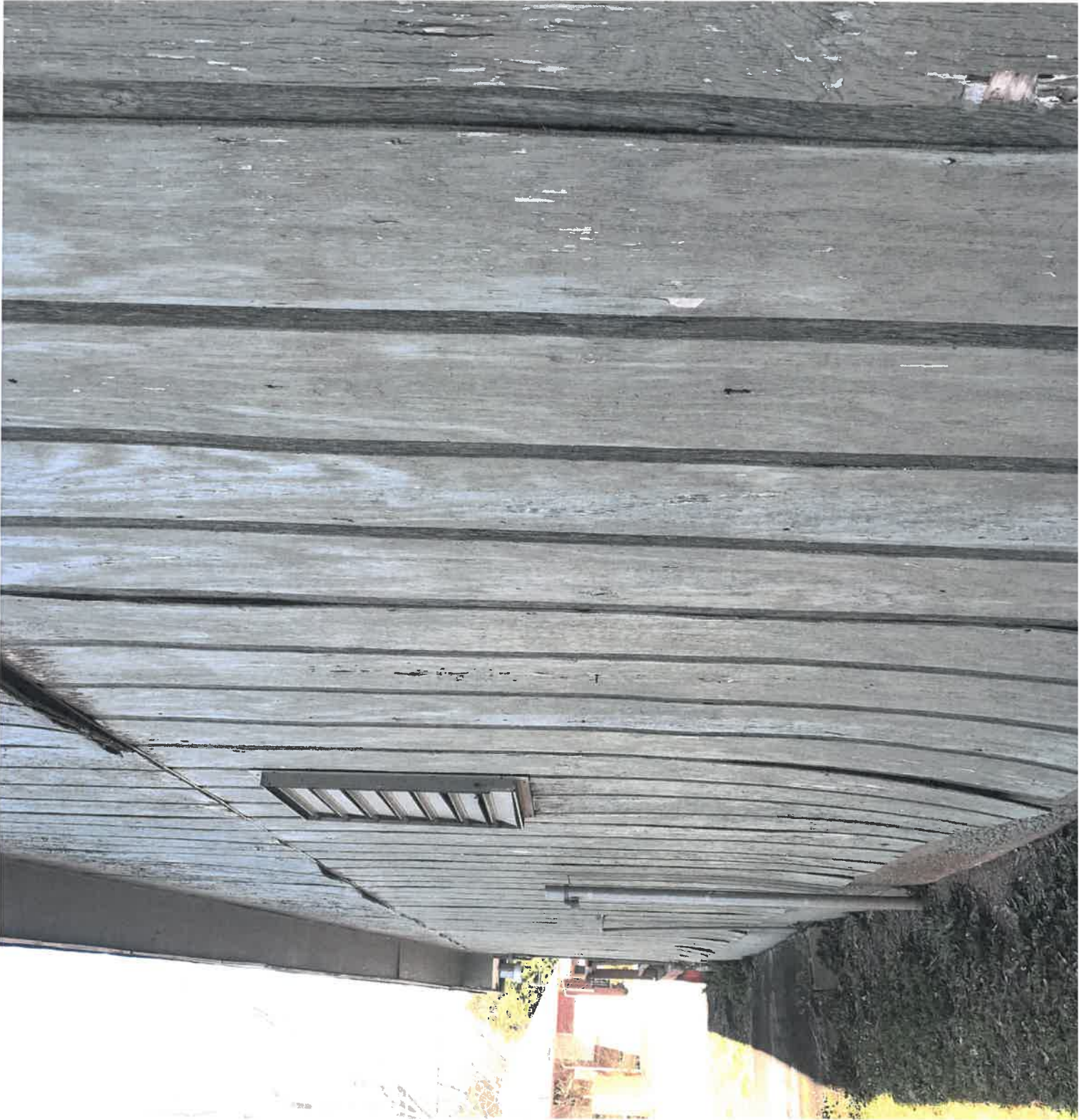
Attachment: Wood Repair (3075 : 234 South Main Street - Bldg Color)
