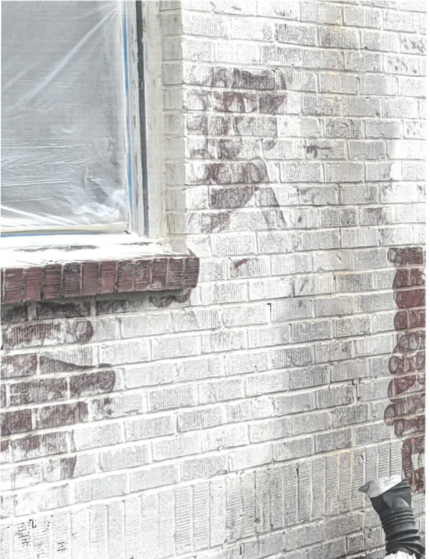
Attachment: Correspondence (3788 : 111 Spring Street - Exterior Brick)
