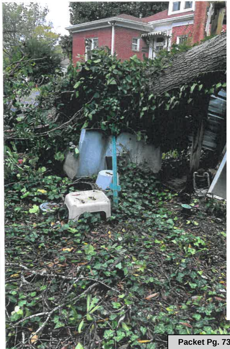
Attachment: Storm Damage (1861 : 145 College Street)
